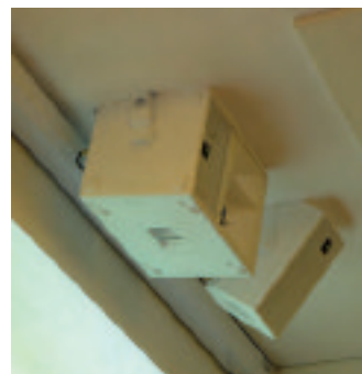
The KV2 Audio ES1.0 and ESD10 speakers recessed into the ceiling
